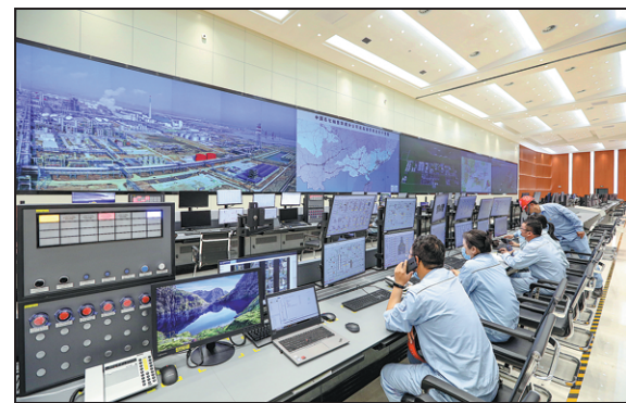
A team of workers keep watch over the control panels of the Zhongke Refinery and Petrochemical project. ZHANG FENGFENG / FOR CHINA DAILY
