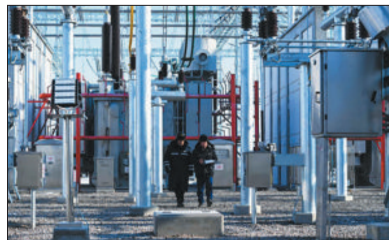
State Grid employees inspect equipment at a power station in Xilin Gol League, the Inner Mongolia autonomous region, in December. PENG YUAN / XINHUA
