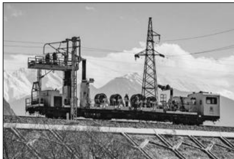
A construction crew sets up electrical lines for the Lhasa-Nyingchi railway in the Tibet autonomous region in February. The line is expected to open at the end of this year. REN FUYANG / XINHUA
