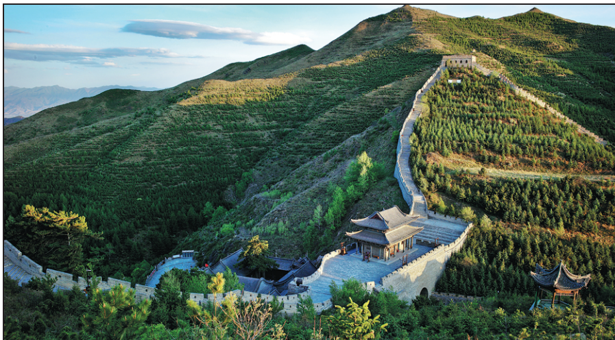
A section of the Great Wall is restored according to its original style. YANG JIANMIN / FOR CHINA DAILY
