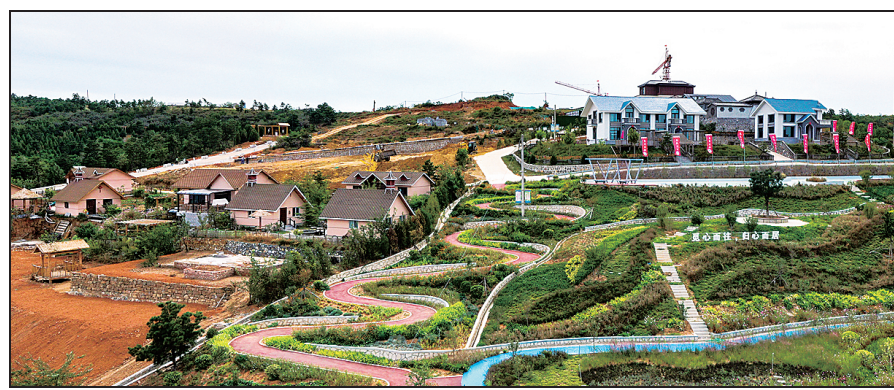
A recreational tourism project is under construction in Wuwangshan village in Jincheng city. NING SHAOXIONG / FOR CHINA DAILY
