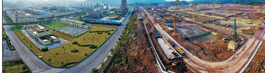
The second phase of the polycrystalline silicon production base under construction in Leshan, Sichuan province, is built by Shanxi Construction Investment Group. YANG YANCHAO / FOR CHINA DAILY
