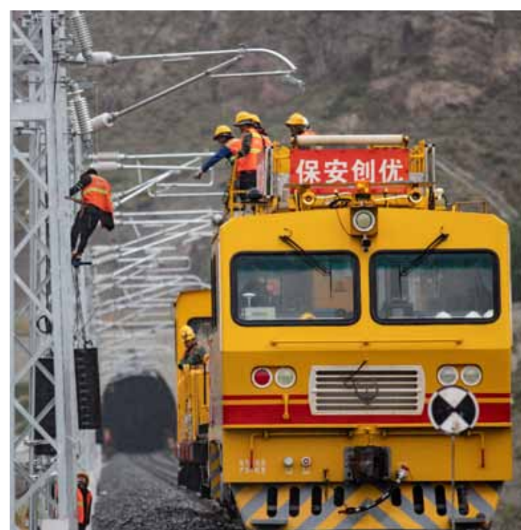
Workers install an overhead catenary system for the Lhasa-Nyingchi electrified railway in mid-August in Sangri county, Lhokha city, Tibet.
