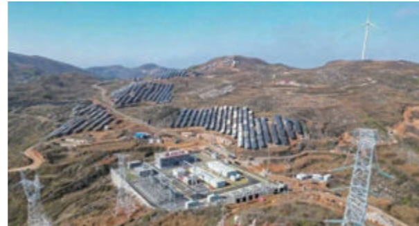
The first batch of square arrays of Ecological Treatment 1 million kilowatts PV Demonstration Project in Loudi, Hunan Province was combined to the grid
