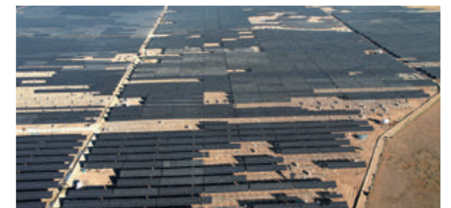
In December 2022, the first batch of photovoltaic modules of the 120,000-kilowatt photovoltaic power supply guarantee project were connected to the grid in Senji District, Nagqu County, Tibet
