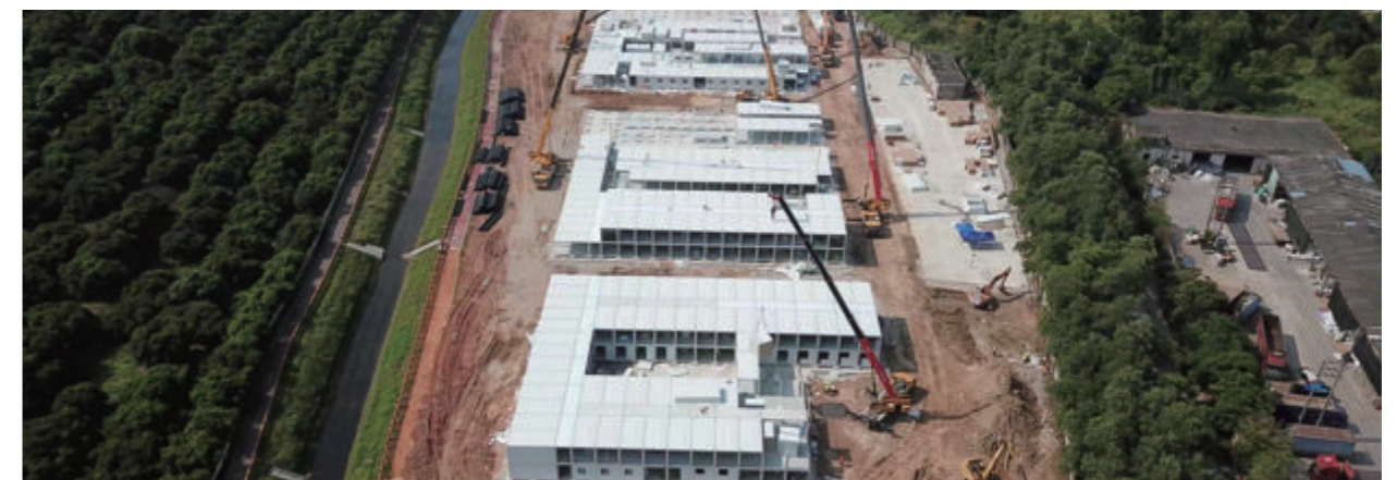
CSSDI participated in the special rectification work for the safety of self-built houses in Hunan Province
