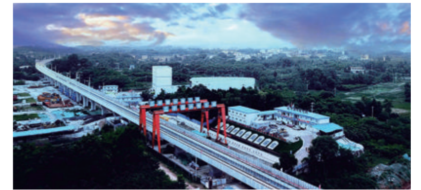
Panoramic View of Track Laying Base of Chengdu Metro Line 18 Track Section 3
